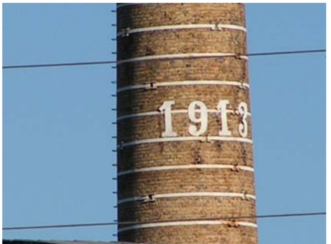
This inscription on the pipe of the sugar factory seems to defy the predominant interpretation of major historical events. It is often stated that such events as World War I or World War II had a huge impact on various local landscapes. It seems that in Rybnitsa these major events are too contentious and locals prefer to celebrate an event which happened in the relatively peaceful 1913.
